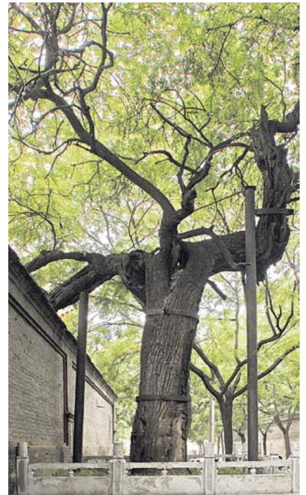
Although not that common in North America, banding trunks and limbs to prevent them from breaking apart is another useful technique and widely seen in China and parts of Europe. Julian Dunster took this picture of a banded Sophora tree in Xian, China.
